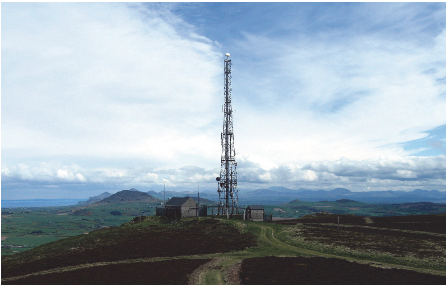
^ Typical customer antenna installation
